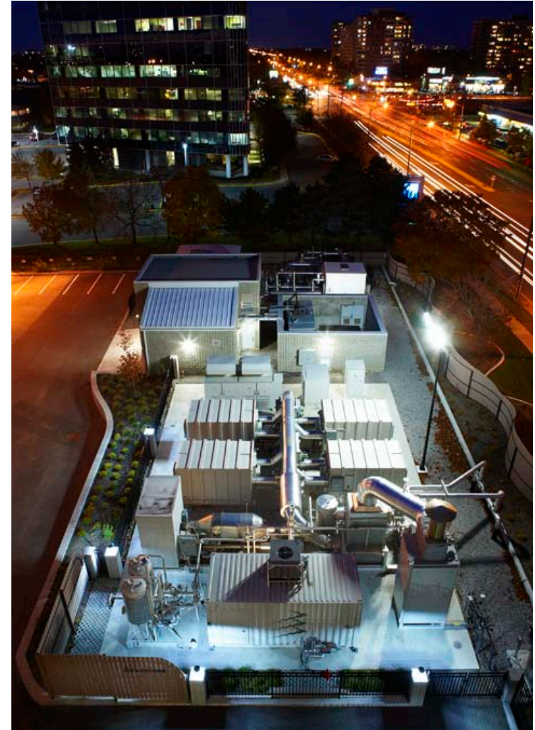
Hybrid FuelCell @ Enbridge's Toronto Facilities
